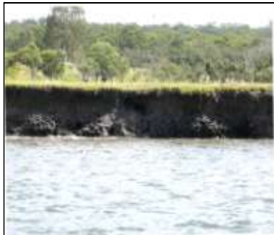
Removal of trees and other vegetation from the banks of the Logan River has resulted in the serious erosion issues evident in the picture at left, taken several kilometres upstream from the bay.
